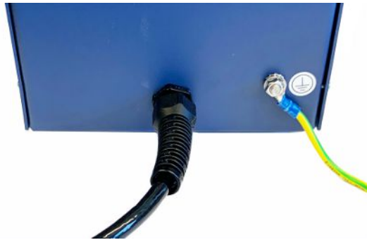
Fig. 2: The grounding strap (here yellow-green) must be attached to the protective earth connection of the interface box!
